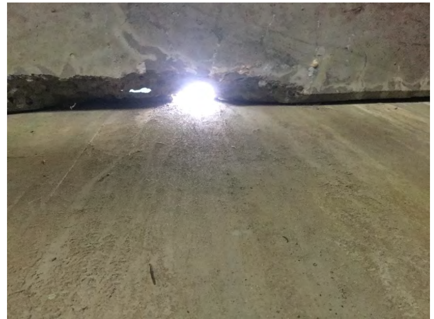
Damage noted on bottom side of panel 1 right bank
