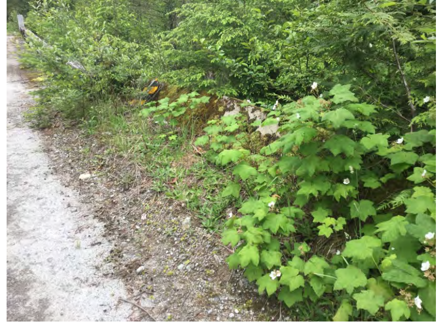
Downstream right bank no posts pushed off road slightly
