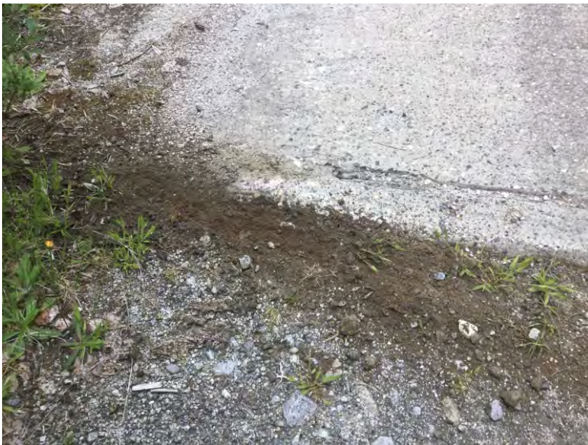
Damage noted to right ballast wall
