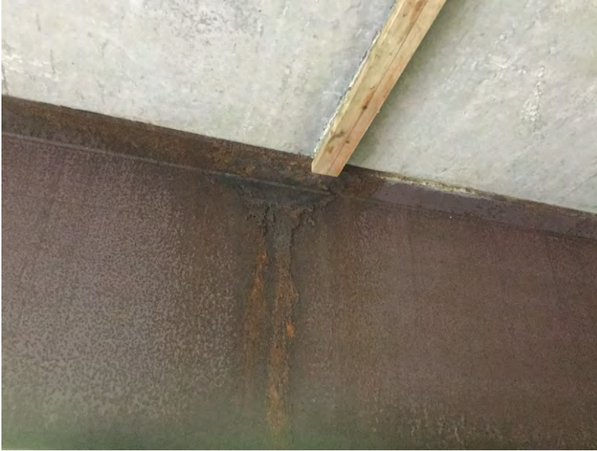
Some water getting through deck joints
